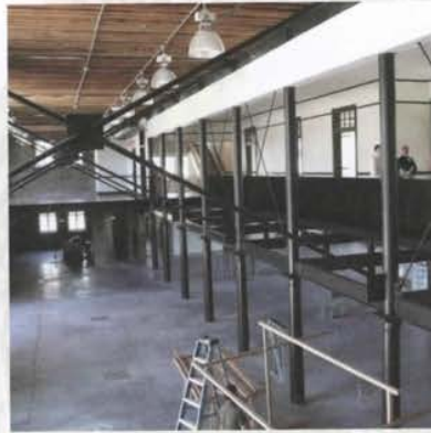
A fresh produce market will be located in this double height space in the former German Schoolhouse, which will also provide offices, R+D facilities and small business incubation units.
